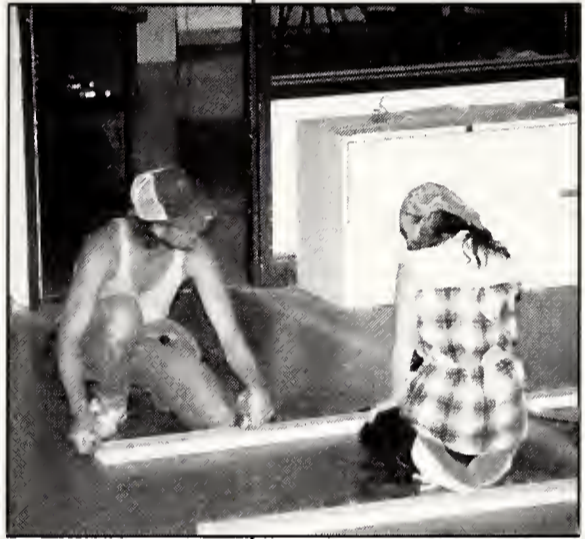
Mrs. Agnes Benson and Mr. Daniel Benson are measuring beams for structure support.
