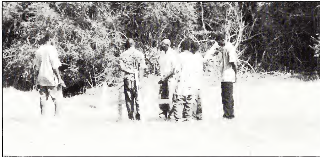
Instructor Mr. Leonard Knight and his class begin by staking out the foundation system.
