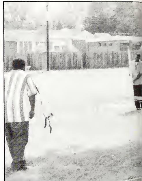
Checking the foundation system for transit are Detrell Brinkley and Denauldo Bennett. Using the leveler are Kamala Banks and Gerald Bradley.
