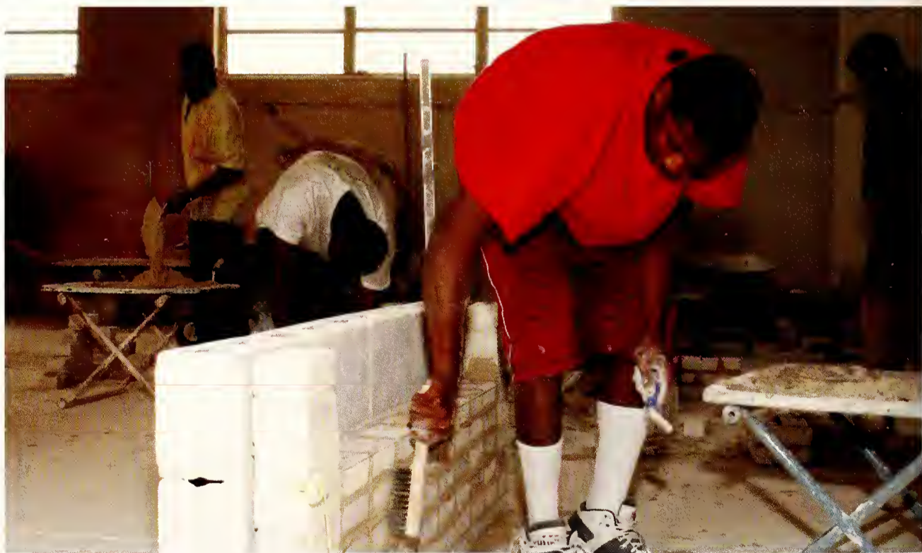
Edwin Gaskin has joined his project and brushes away excess mortar for a finished product.
