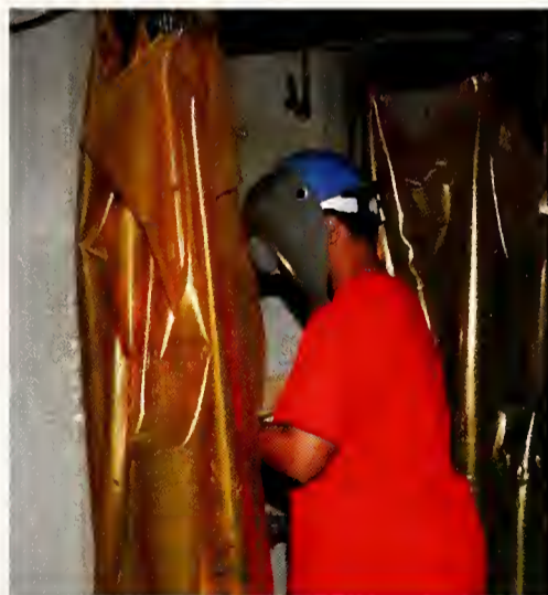
(above) Brandon Dent finishes a rod welding project and cleans his metal.
