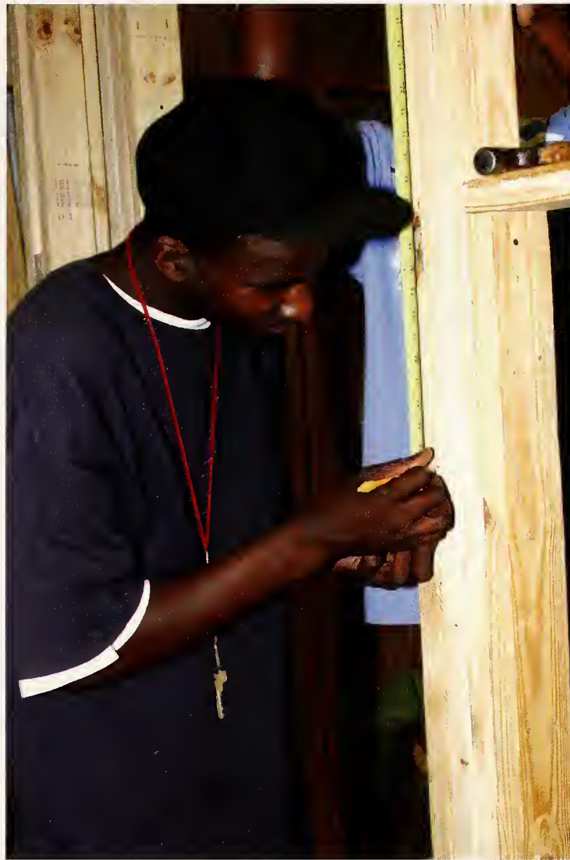
Left: Ricky Hearn marks the height for a door installation on a model house.
