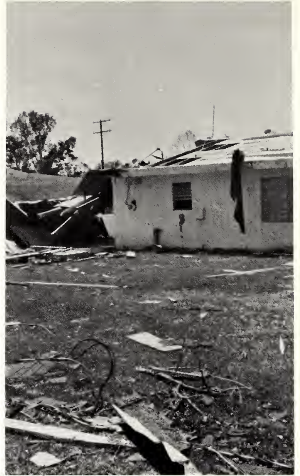
Rear structural damage.
