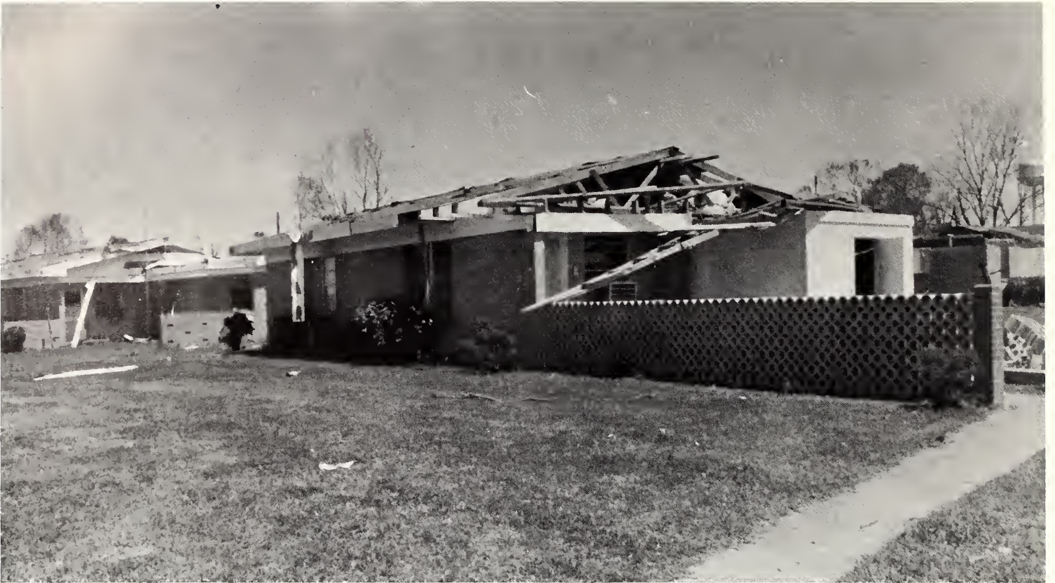
A house damaged by the tornado.
