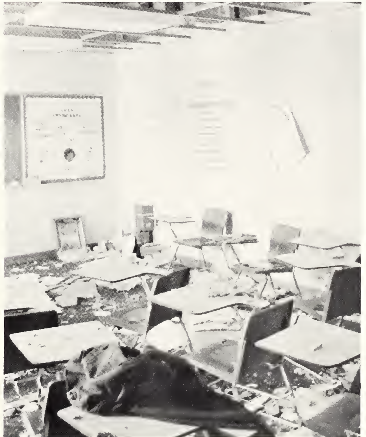
A damaged classroom.
