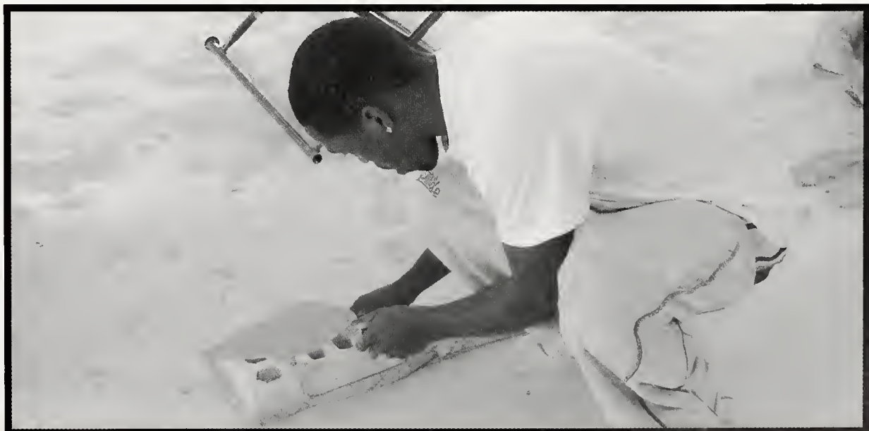
A student applies cement to a series of bricks in preparation for a foundation of a project on which he is working.
